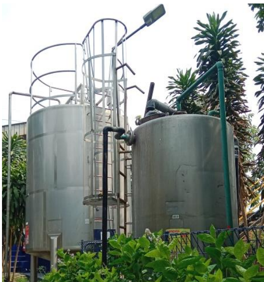
Gambar 4. 6 Spare Tank di WWTP (Sumber : PT Tirta Investama (AQUA ) Pandaan)
