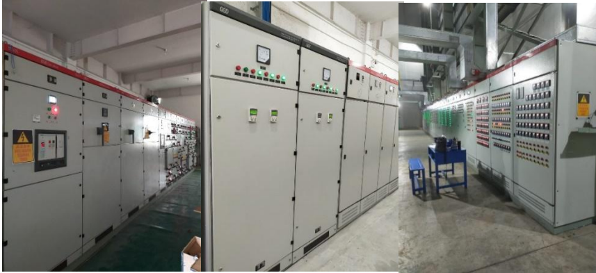
Gambar 1.1 Panel Distribution Control
